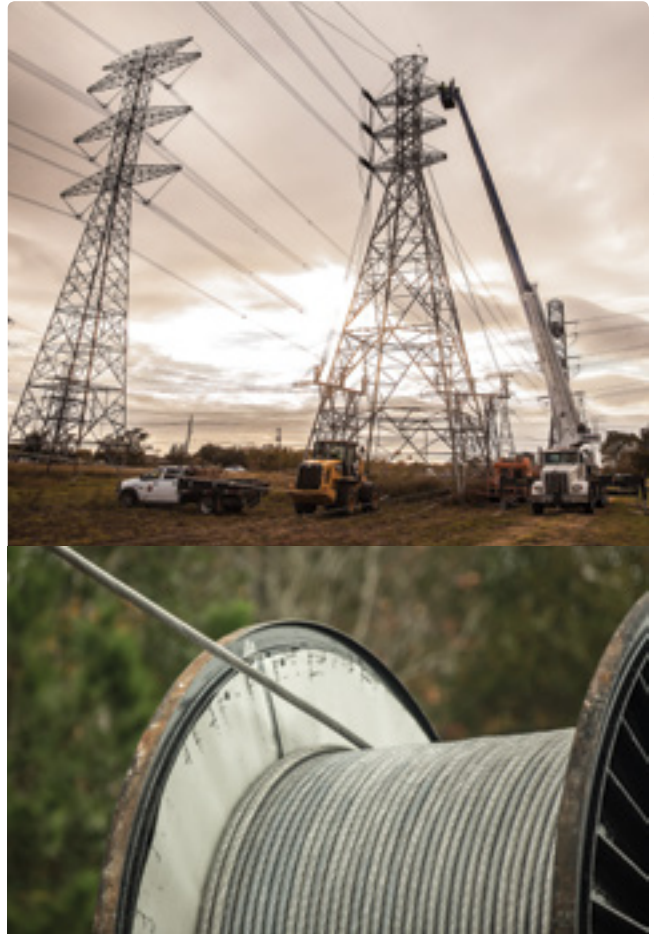
Source (both photos) | Celanese/Southwire
