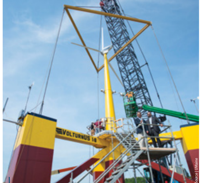
The VoltturnUS ' patent-pending concrete semisubmersible hull design can be seen here, prior to the floating turbine system's launch. ■
